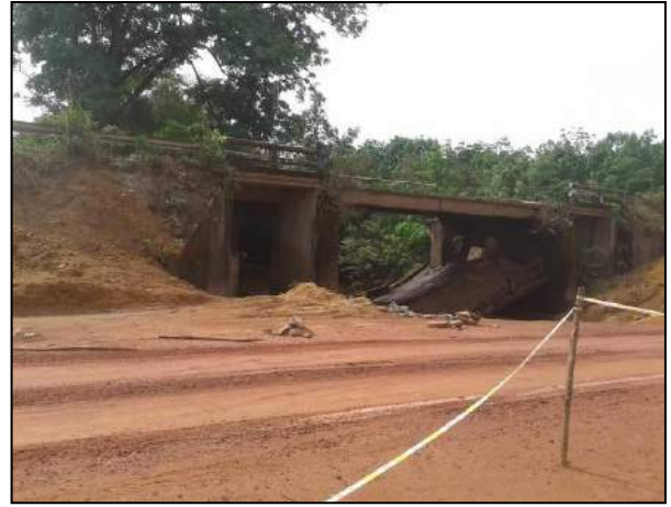
Figure 3: Destroyed Bridge Structure
