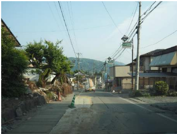
Figure 10. Pavement peeling at Mashiki Town
