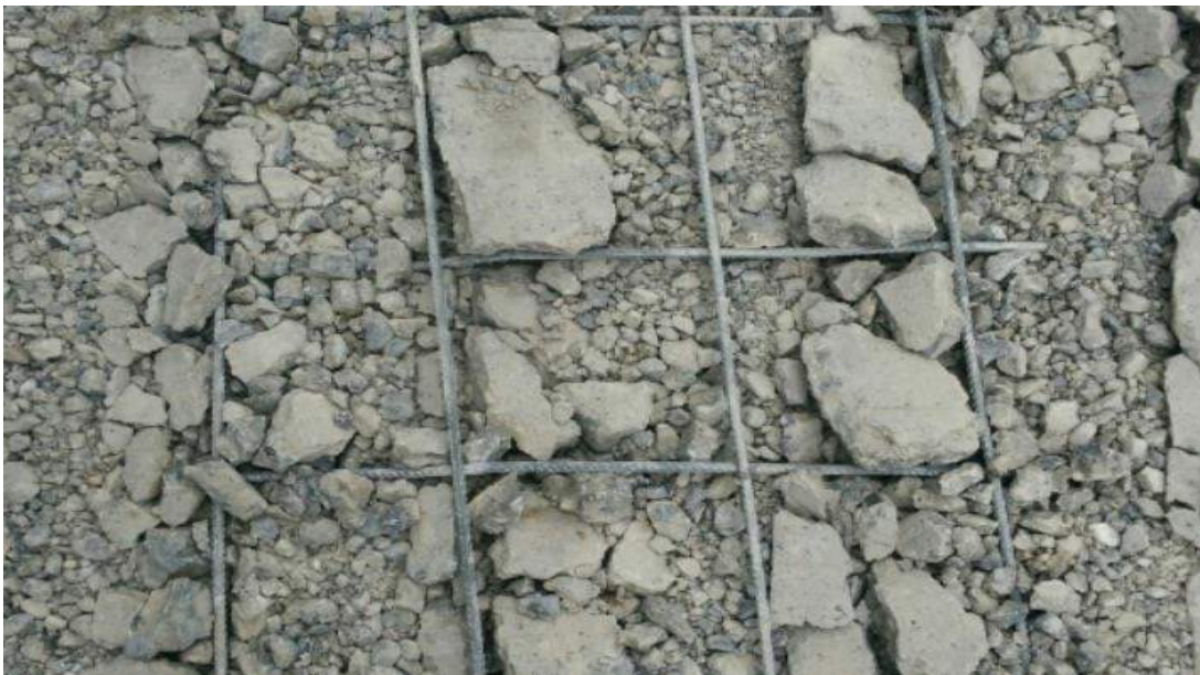
Figure 3. De-bonded reinforcing bar after rubblization.
