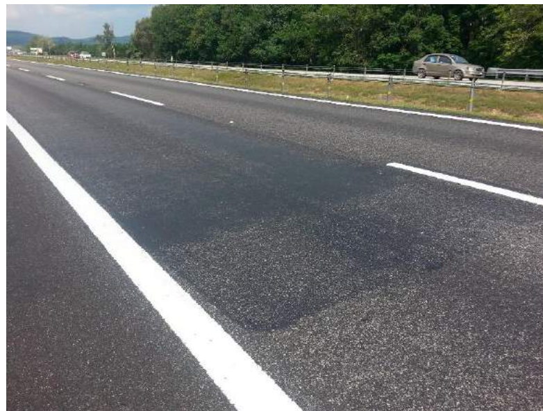
Figure 4b. Poor surface texture
