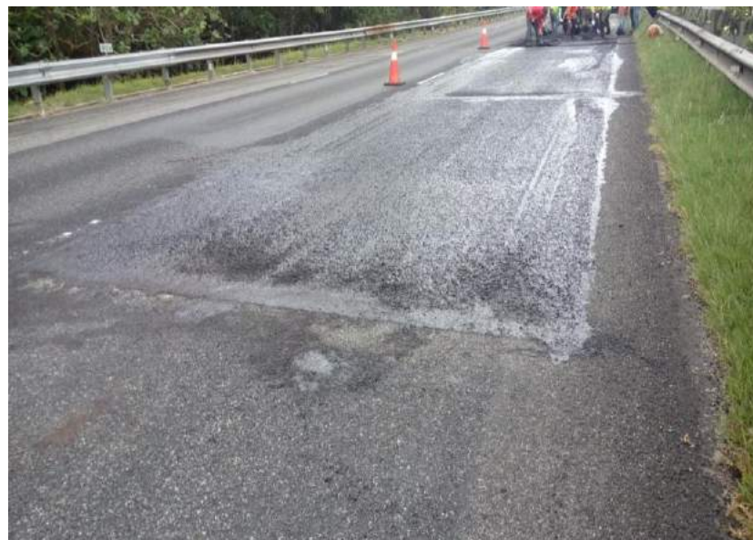
Figure 3b. Poor quality transverse joint
