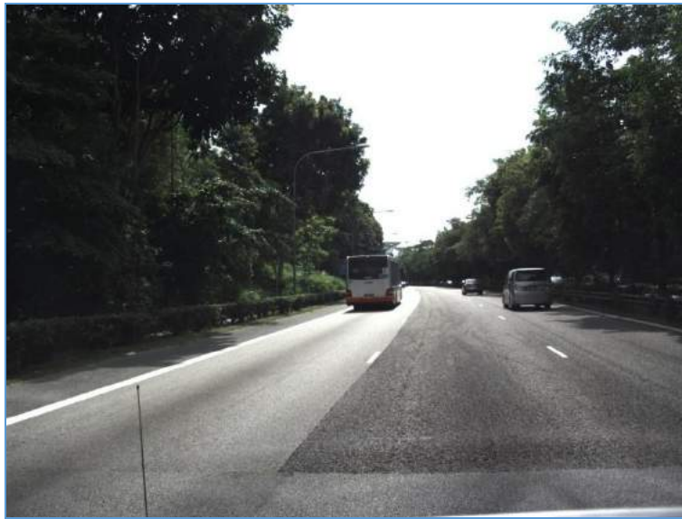
Figure 4. Observed raveling Expressway Singapore
