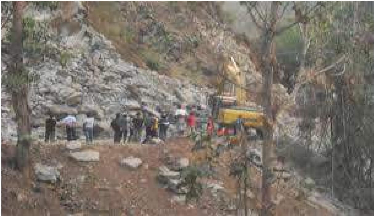
Figure 3. Avalanched Debris Falls at KM 76+000 Ende, Trans Ende – Maumere East Nusa Tenggara Province, Indonesia (IRE, 2008)
