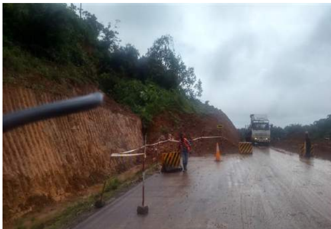
Figure 14: An Earth Batter Failure during Construction
