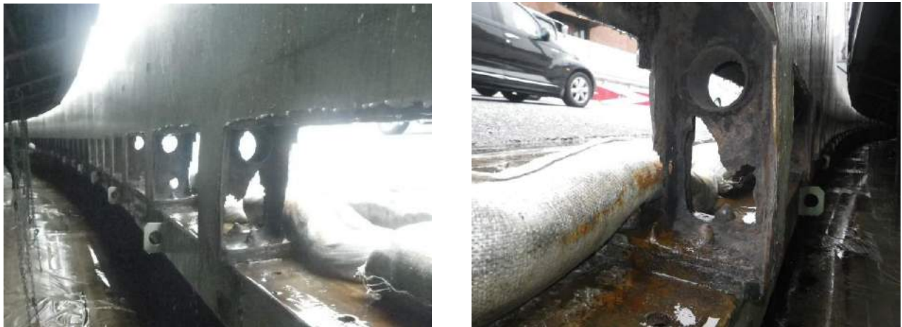
Figure 1.Reduction of Cross-sectional Area due to Internal Corrosion of Steel Barrier Posts
