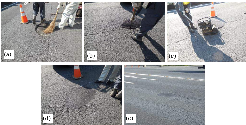
Figure 11. Work procedure for pothole repair material: (a) Cleaning, (b) Unpacking and spreading/leveling, (c) Compacting, (d) Completion, and (e) Traffic opening
