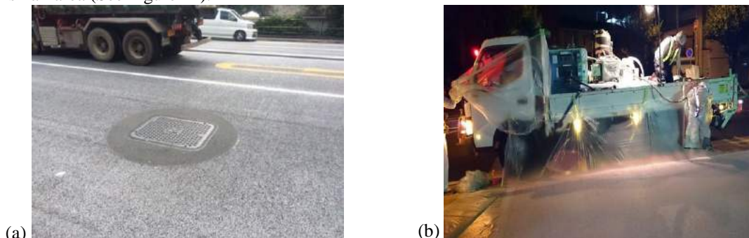
Figure 11. Small scale repair and conventional application train (a) repair area, (b) application machine
