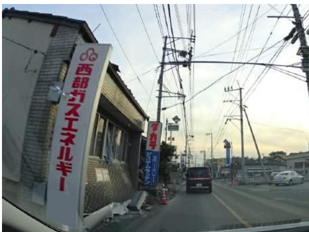
Figure 8. House collapse at Mashiki Town
