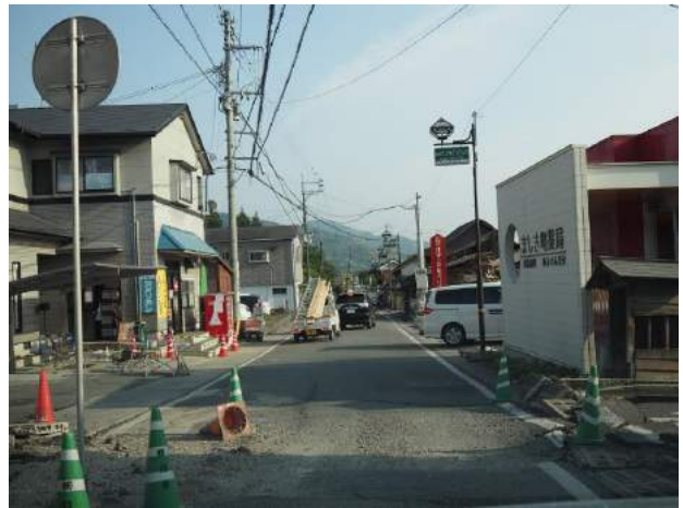
Figure 11. Pavement peeling at Mashiki Town
