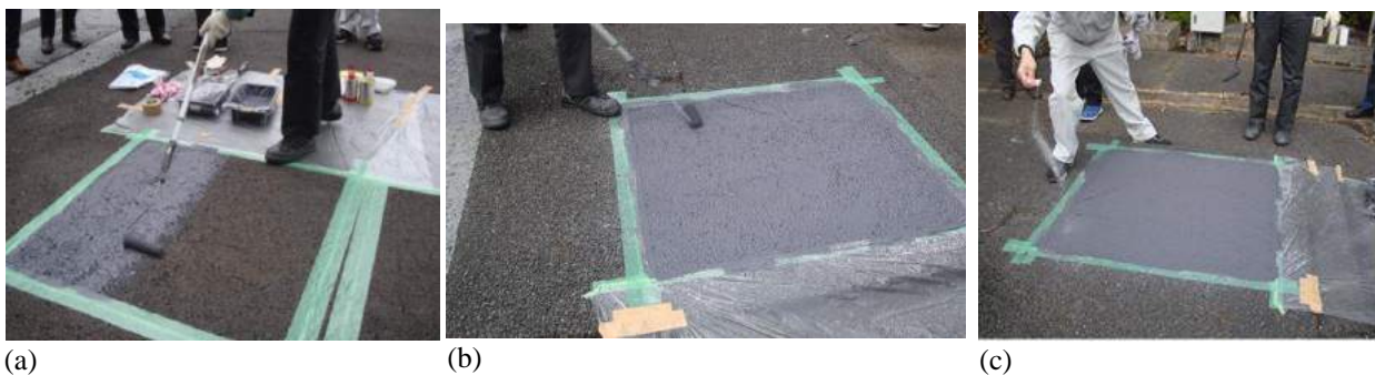
Figure 13. Application of the repair kit (a) Application of 1 st layer, (b) Application of 2 nd layer, (c) spray non-skid sand.
