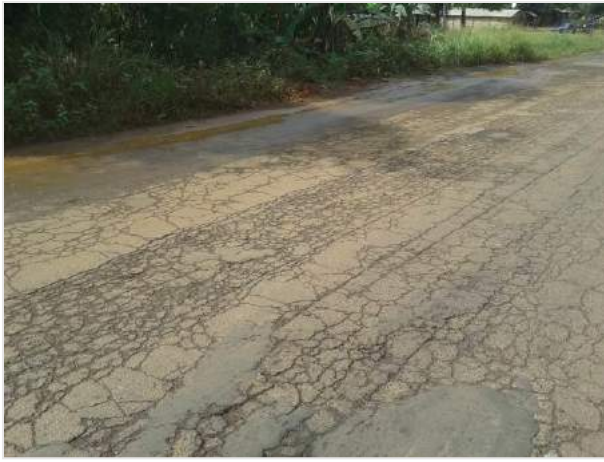
Figure 2 Existing Pavement – Pre-rehabilitation.
