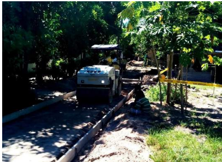
Figure 4. Compaction of subgrade with mechanical roller. Note edge beam formwork in place.
