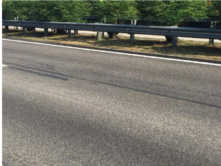
Figure 5. Dragging line on micro surfacing surface.
