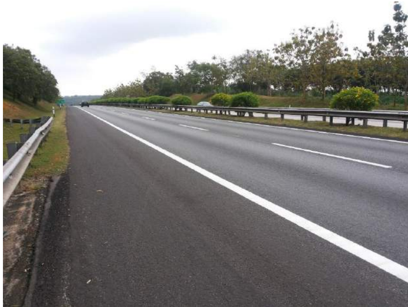
Figure 2a. Good quality longitudinal joint.
