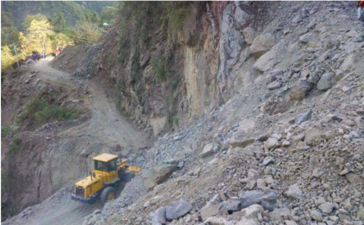
Figure 5. The Evidence of landslide at other side of KM 17+000 Ende during road widening progress, East Nusa Tenggara Province, Indonesia (Tribun News Kupang, 2013)
