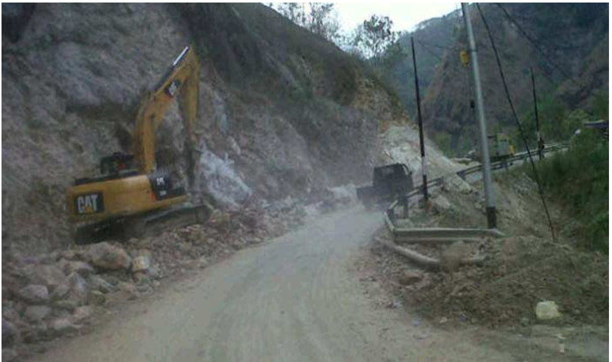
Figure 4. Landslide Evidence at KM 46+000 Ende, East Nusa Tenggara Island, Indonesia (Pos Kupang, 2016)
