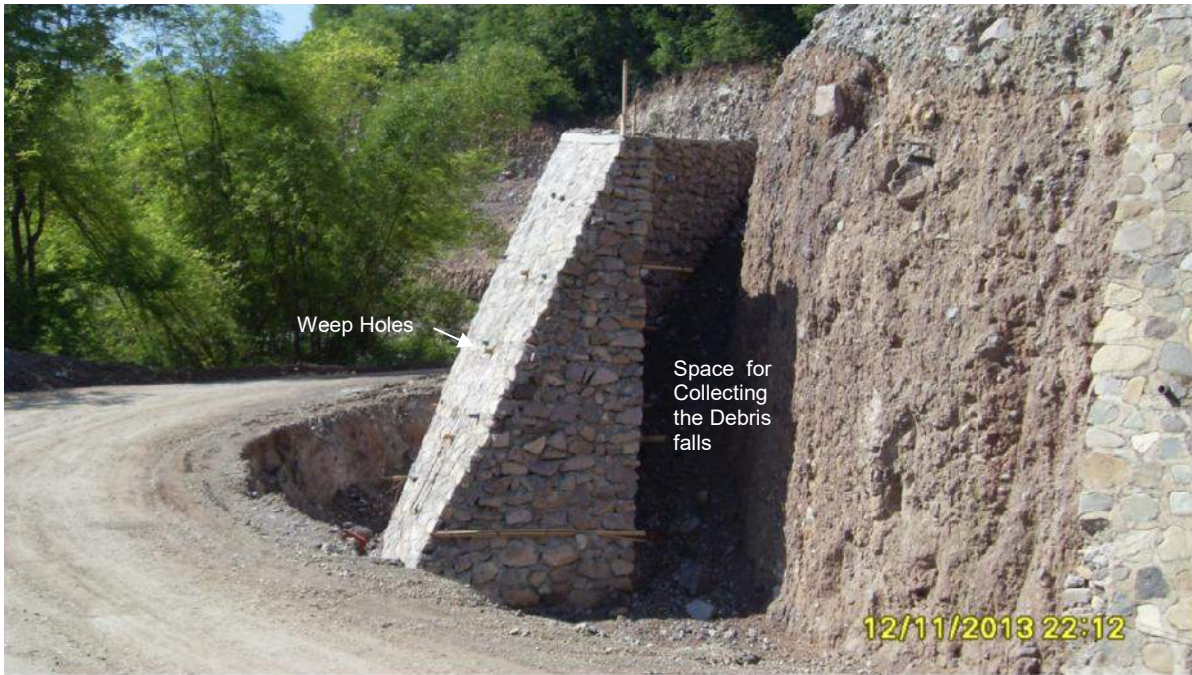
Figure 8. Implementation of Fence Defense as Earth Retaining Structure at KM 17+000 by local Government Authority (IRE, 2013)
