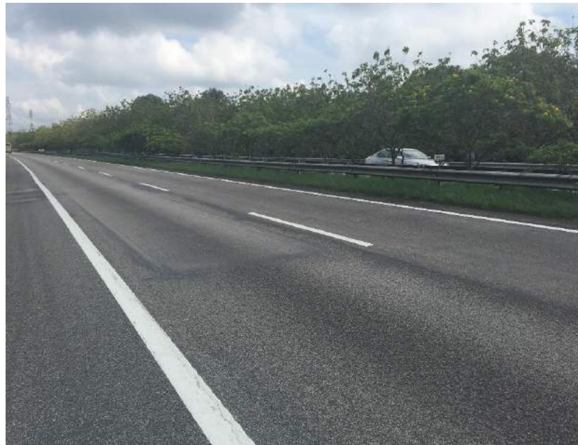
Figure 2b. Longitudinal joint on wheel path and excessive binder on joint.
