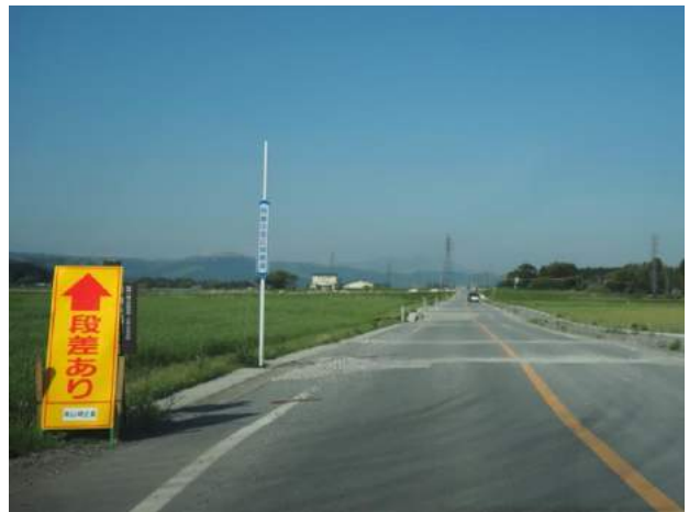
Figure 13. A bump step sign at Aso City
