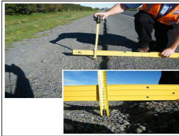
Figure 15: Example of a Shoulder Drop-off Defect and Measurement Method
