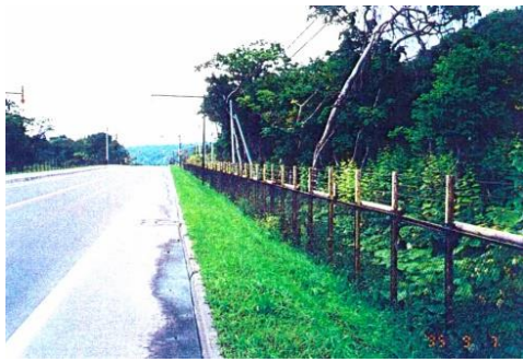
(a) 侵入防止柵
